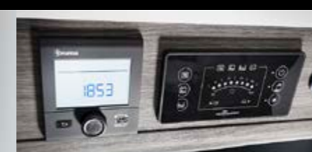
15 Onboard control above the sliding door
