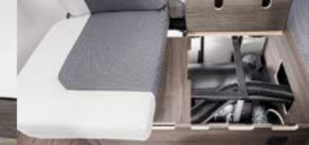
4 Diesel heating in the living area
